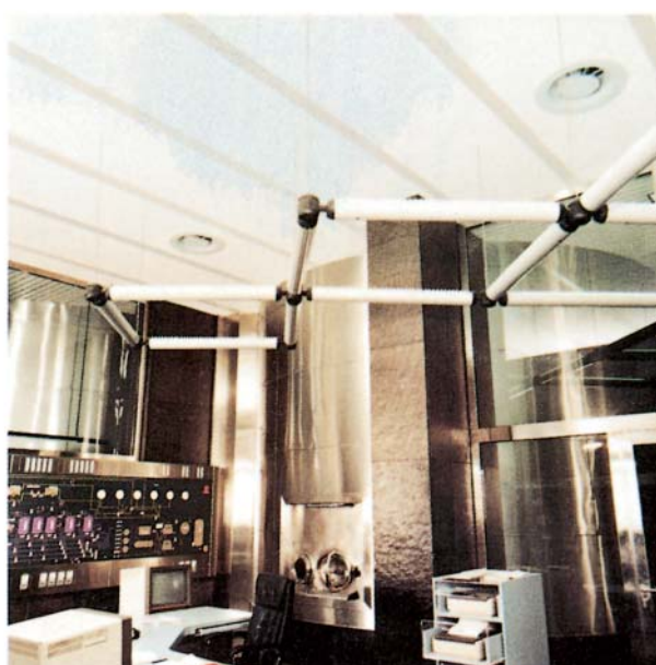
Control room: König Brewery, Duisburg
